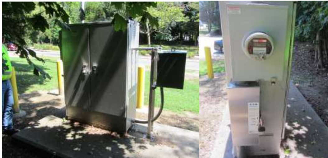
Existing Electrical Service Cabinet
